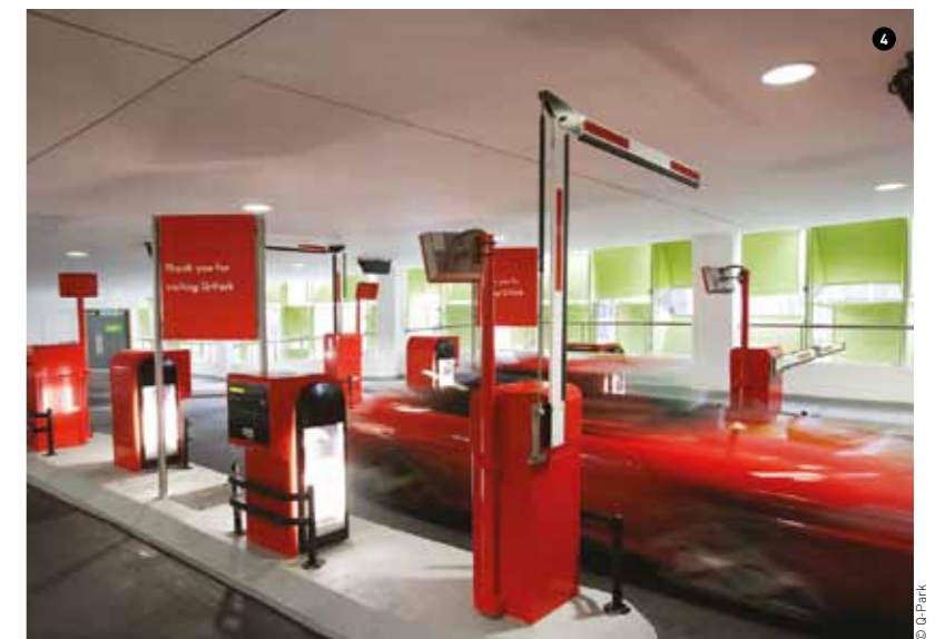
3 Q-Park, Sheffield, England Energy savings are instant, with luminaires being active only when needed. 4 Q-Park, Sheffield, England LED luminaires can be programmed to dim after a period of inactivity.
